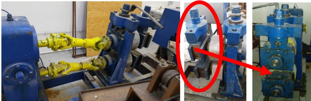
Fig. 2. a) Rolling mill overview; b) Roll stand without one pillar; c) Missing part positioning.
